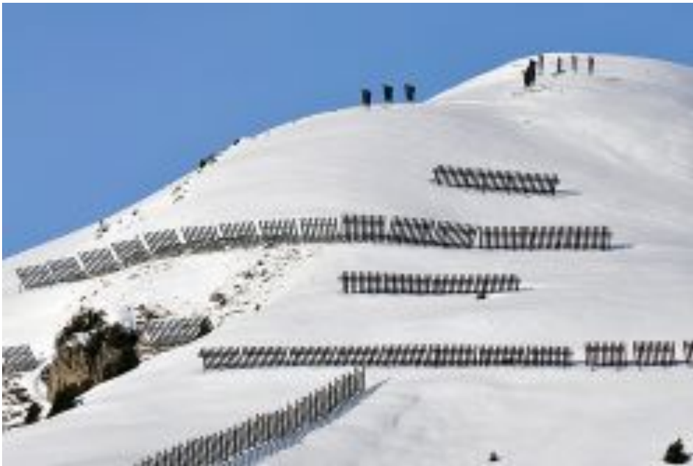
Fences for stabilizing snow
